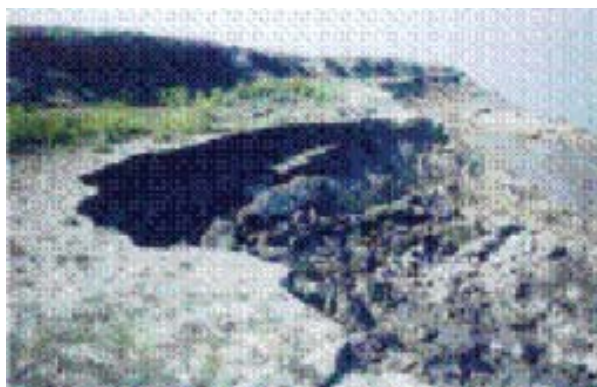
Fig. 6 : River Bank Failure of the Brahmaputra River at Neamatighat, Jorhat District, Assam
